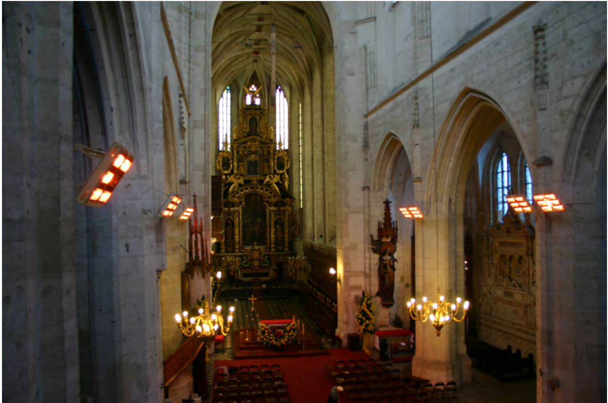
Fig. 4. Main nave of church of St. Catherine in Cracow, Poland, 1365e1400. Electric heaters, comprising six radiant tubes each, are mounted permanently at a height of 7 m above the floor.
