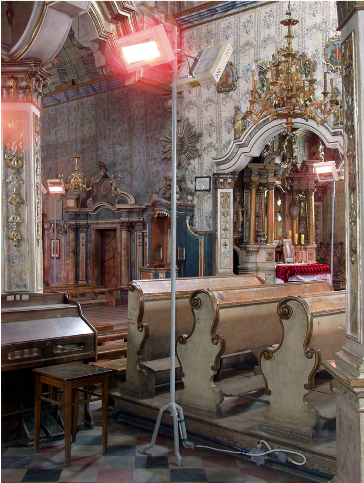
Fig. 3. Details of mounting the heaters on the metal rods at the height of about 3.5 m above the floor.
